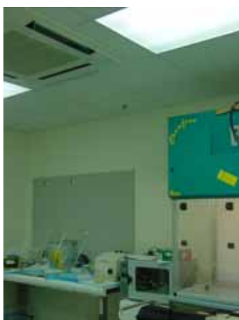
Figure 4: Supply air from the air conditioner installed on the ceiling affected the performance of fume cupboard.
