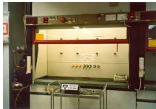
Figure 2: An auxiliary fume cupboard with supply air from the two sides behind the sash.
